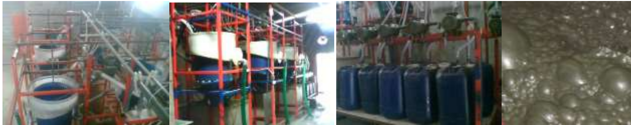
Copper Extraction Plant installed in East Java
